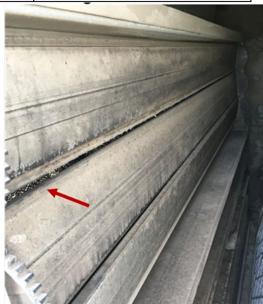
Figure 3. Picture of a warped damper blade unable to close.
